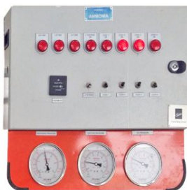
Pressure cutout PLC Panel
